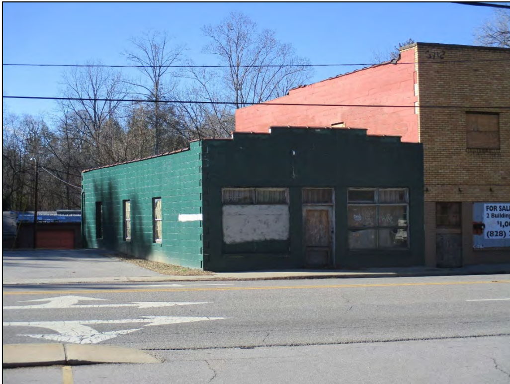
Former Keith’s Super-Cleaners oblique view of façade and south elevation, looking northwest
