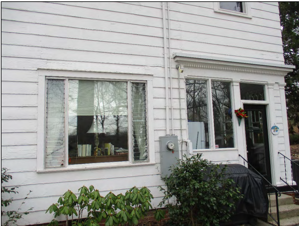
Rhodes House rear (west) elevation picture window and enclosed porch (at right), looking southwest
