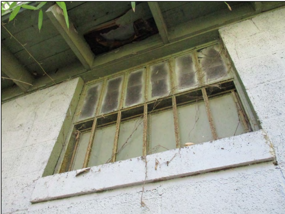
Former Morrison's Furniture Store rear (east) elevation detail of steel casement windows in the rear lean-to addition
