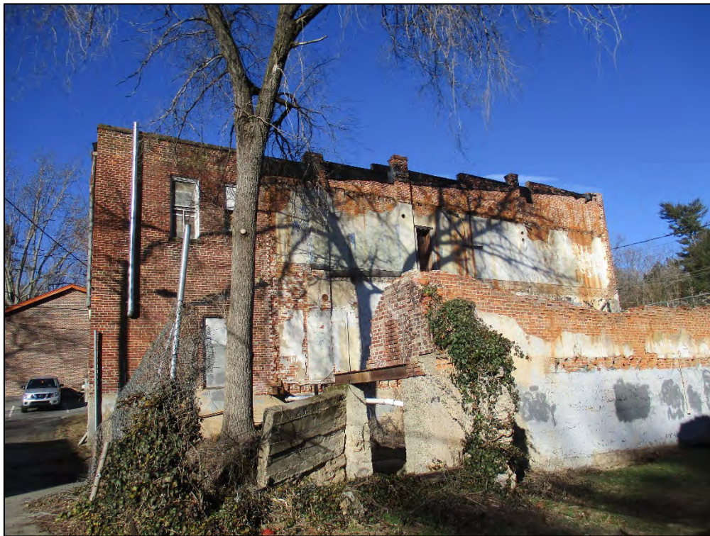
Allison's Grocery, view of exposed south elevation from the alley, looking northeast. The party wall ruins in the foreground are remnants from the three-part building once filling this area.
