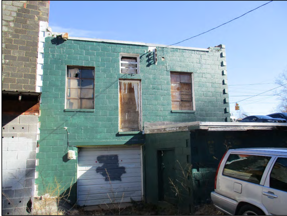
Former Keith's Super-Cleaners rear (west) elevation, view to the west. The former Moser Plumbing Building is visible at left.
