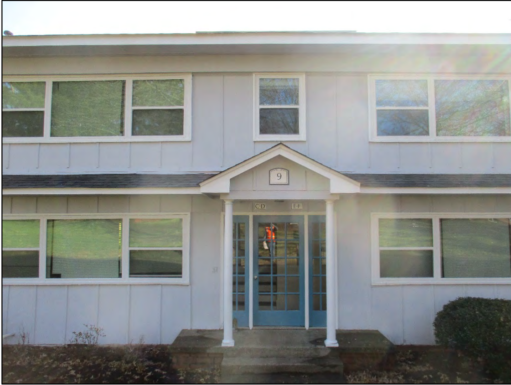
Edgewood Knoll Apartments Building 9 façade garden apartment entry detail, view to west
