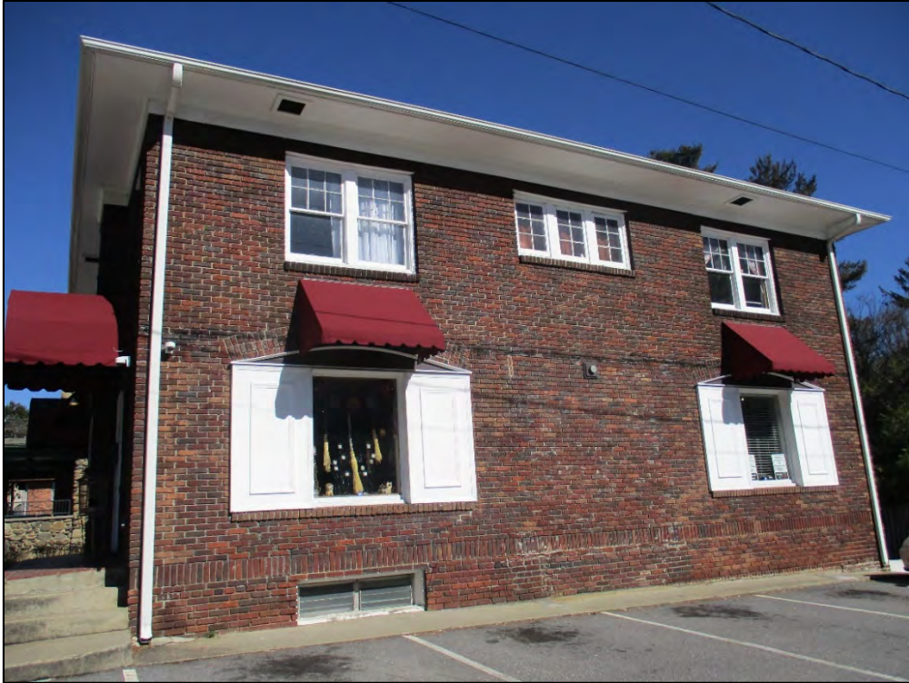
South elevation, facing northeast. Previous survey and current field investigations suggest this elevation originally served as the façade, with a centered entry between the triple windows (see detail below).
