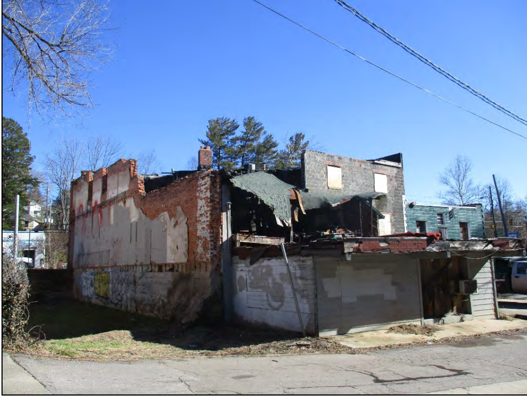
Former Moser Plumbing Building oblique view of the rear (west) and north elevations, view to southwest. The brick wall along north elevation is remnant from adjacent building that has been demolished.
