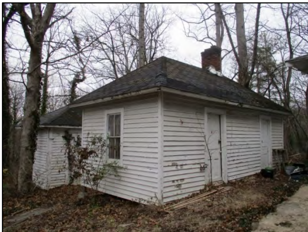
Rhoades House oblique view of servant quarters south and east elevations, view to the northwest
