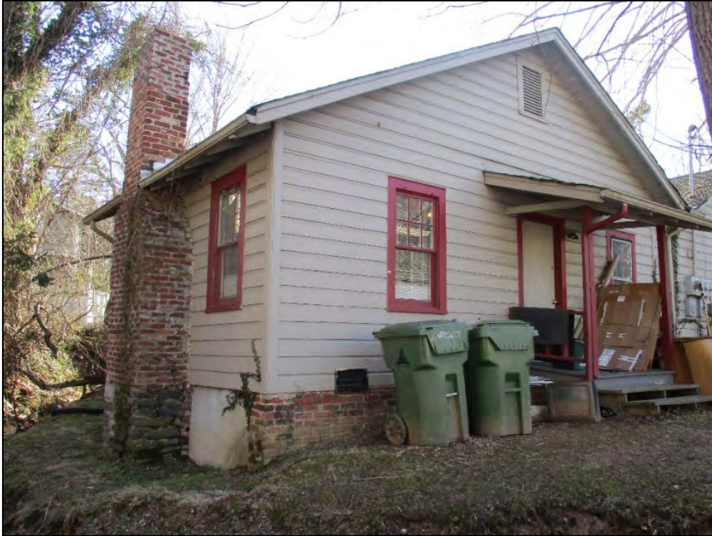
Oblique view of gable addition at northeast corner of house, view to southwest. This addition appears to date to the same period as the additions to the rear of BN5736.
