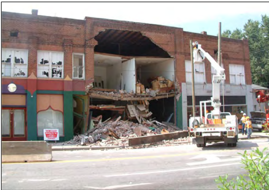
Exhibit 29. 500-502-504 Merrimon Avenue in 2005, following a vehicle collision with the central unit (502 Merrimon Avenue) and the collapse of the façade. This photograph reveals the full extent of the historic construction, a three-unit brick-front with slightly projecting, dominant central mass. Only 504 Merrimon Avenue (BN5742) (at right) remains. Source: Asheville.com ( www.asheville.com/news/merrimon0905.html ).
