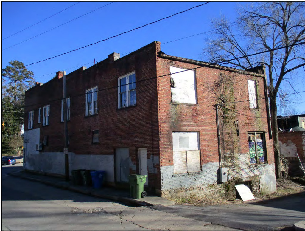
Allison's Grocery oblique view to the southeast of the rear (west) and north elevations
