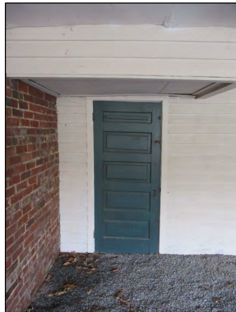
Clearview Terrace Apartments Building B east elevation, converted carport/garage detail, presumed original door and siding, view to west
