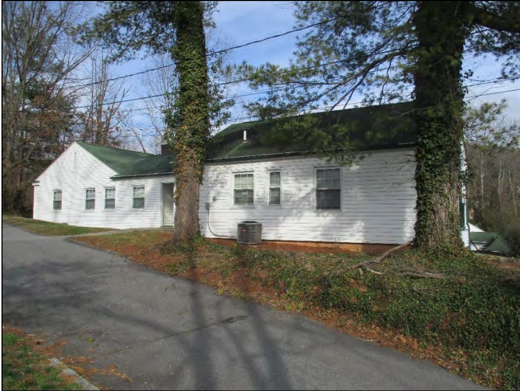
Clearview Terrace Apartments Building B, Units 5 and 6 rear (west) elevation, view to northeast
