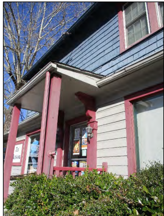
Façade shed portico detail, view to northeast. Note the pilasters and brackets.
