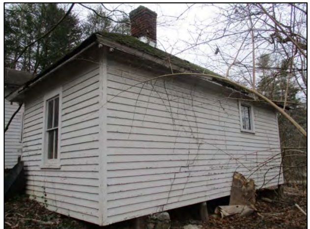
Rhoades House oblique view of servant quarters north and west elevation, view to the southeast
