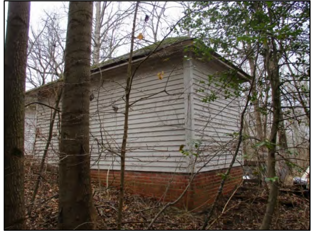
Rhoades House storage shed oblique view of north and east elevations, view to the southwest
