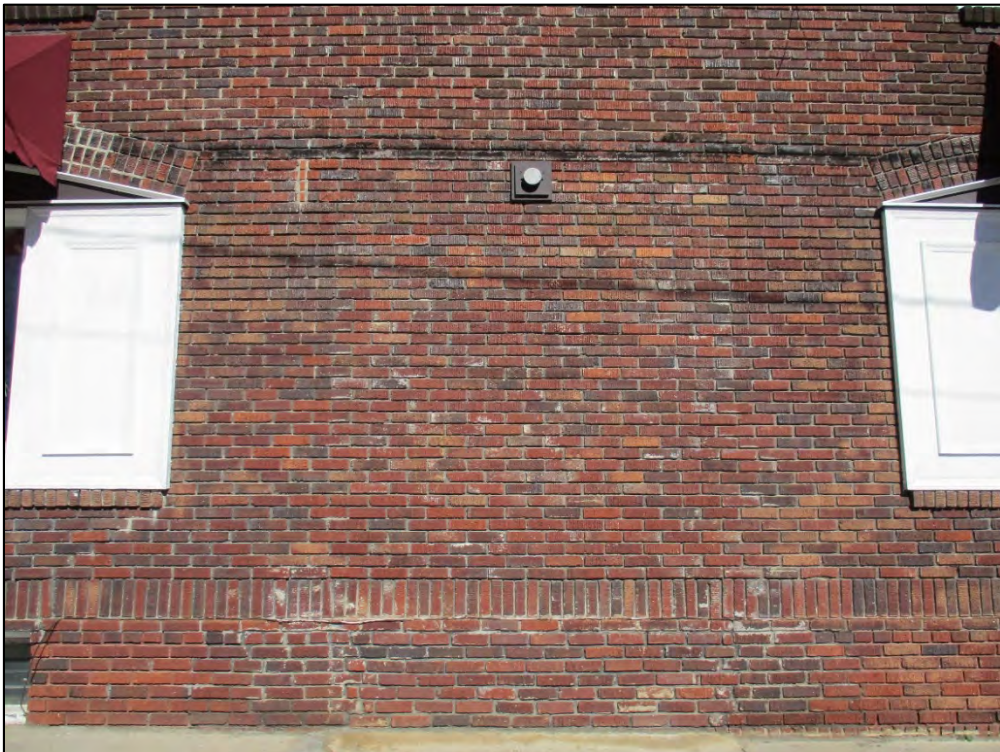
South elevation detail, location of suspected historic entry discernible by mortar treatments and tar line
