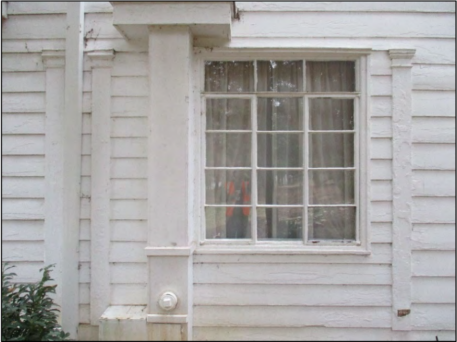
Rhoades House south elevation window detail. Also note pilasters in first story.
