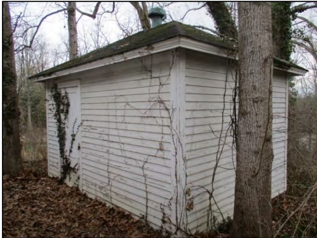
Rhoades House oblique view of Apple Shed north and east elevations, view to the southwest
