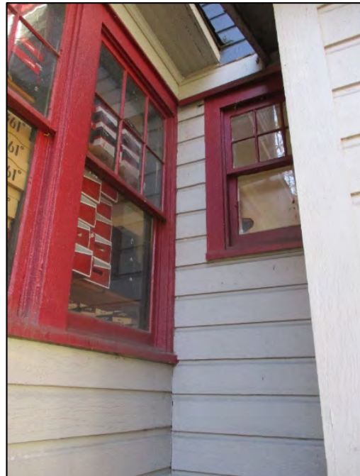
Rear (east) elevation detail of the two-story addition junction, view to north. Note the two-story addition (to the right) partially covers window surrounds (at left) and the boxed eave above.
