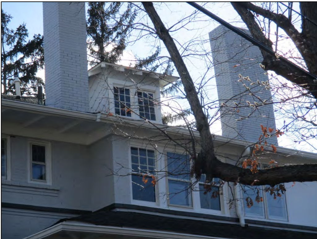
Edgewood Knoll Apartments leasing office west elevation window and dormer detail, view to southeast
