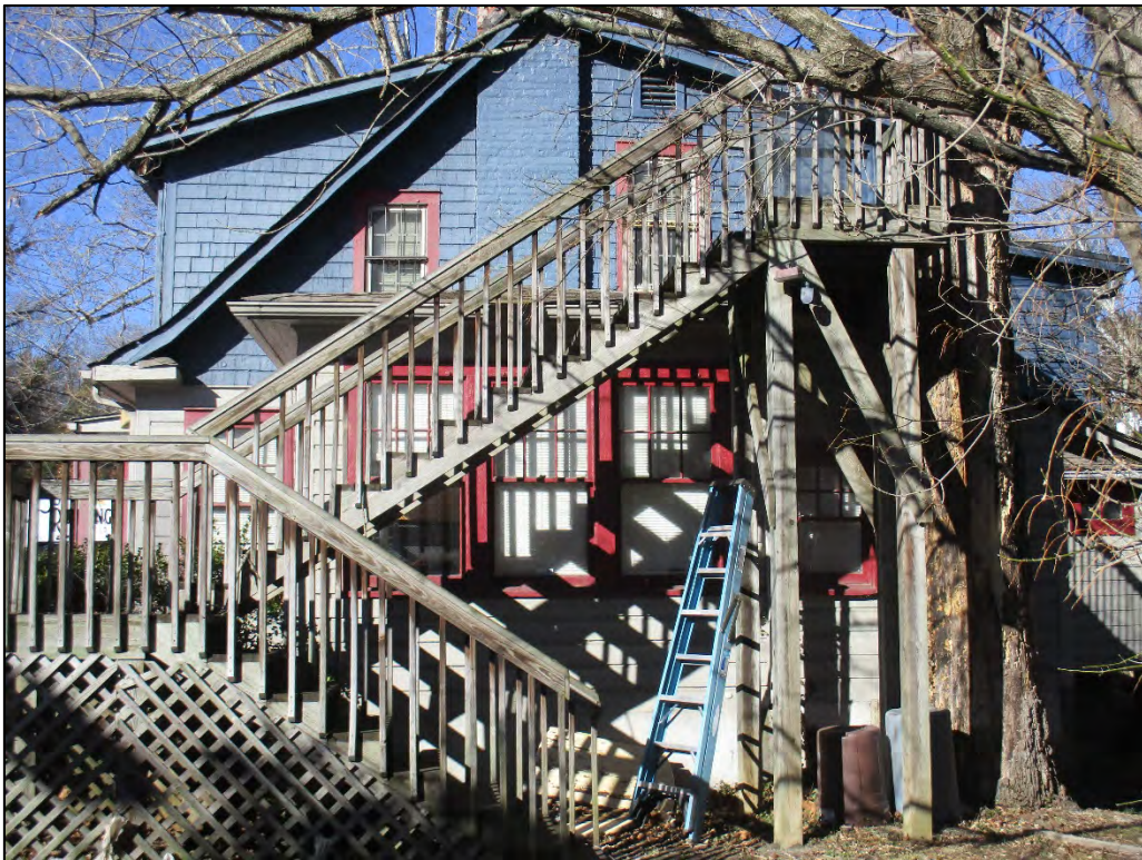
South elevation, view to north. The ribbon of four windows in the hipped roof wing is partially obscured by deck structure.
