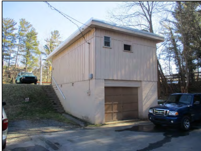
King's Barber Shop oblique view of the rear (west) and north elevations, looking southeast
