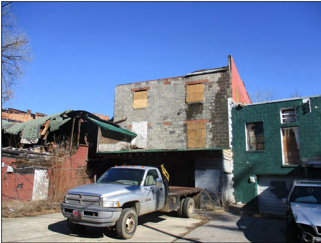
Former Moser Plumbing Building rear (west) elevation, view to the northeast. Keith’s Super-Cleaners is at right.
