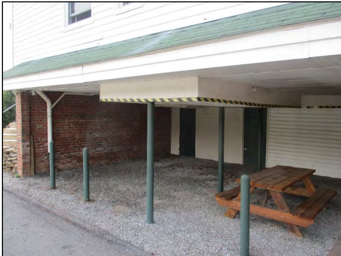
Clearview Terrace Apartments Building B east elevation converted carport/garage detail, view to southwest
