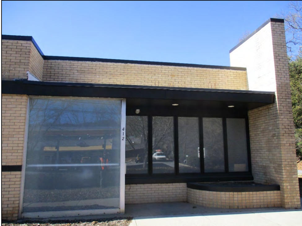
Former Western and Southern Life Insurance Company façade detail of the integrated canopy and altered entry, view to the west
