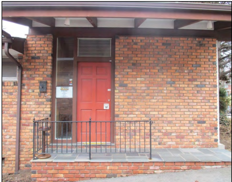
Ray Dental Office north elevation primary entry detail, view to the south
