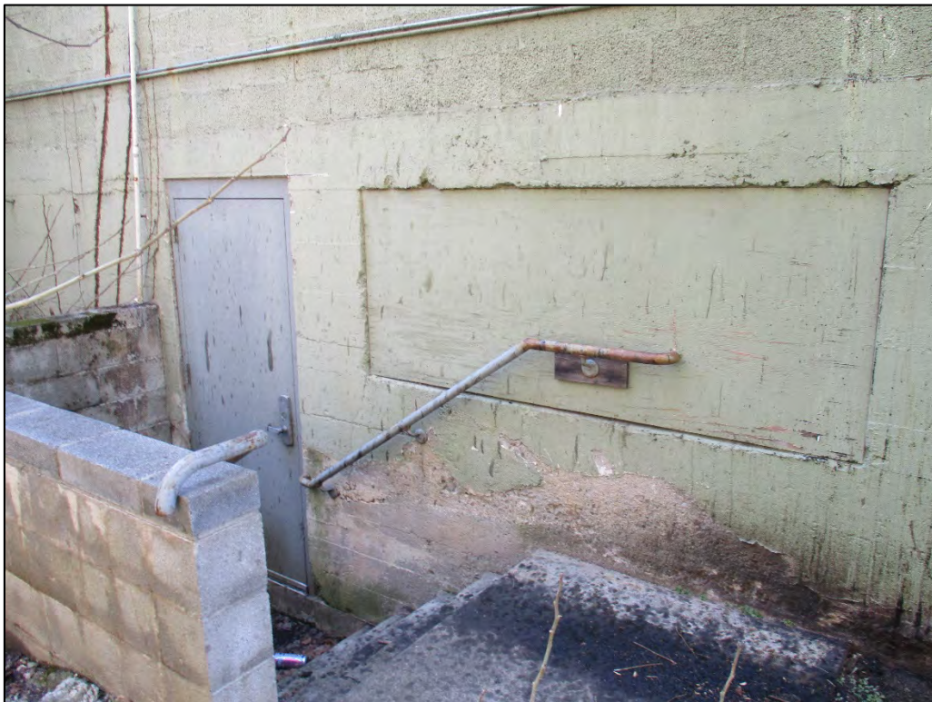
Former Morrison's Furniture Store rear (east) elevation basement door detail, located in the north side of, looking southwest
